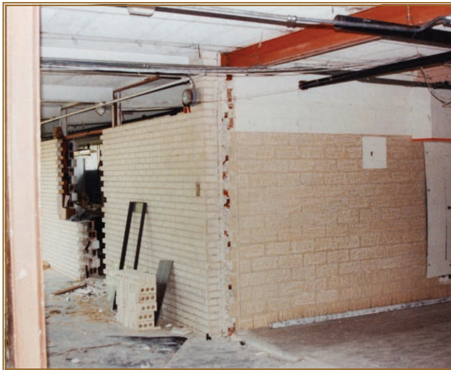
Glazed block and brick in an elementary school renovation about to receive SKIMM™; to be followed by Duroplex® system.
